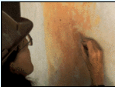
Microorganisms have caused this stain to appear on a marble column at the Jefferson Memorial.
