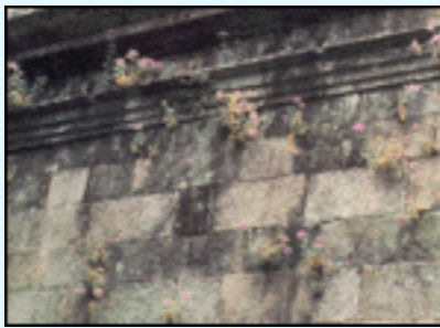
Flowers and grasses have grown in the cracks between stones on this church.
