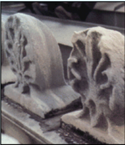
When marble is exposed to acidic rain, sharp edges and carving details gradually become rounded. Antefixes, roof of the Philadelphia Merchants' Exchange (built in 1832).
